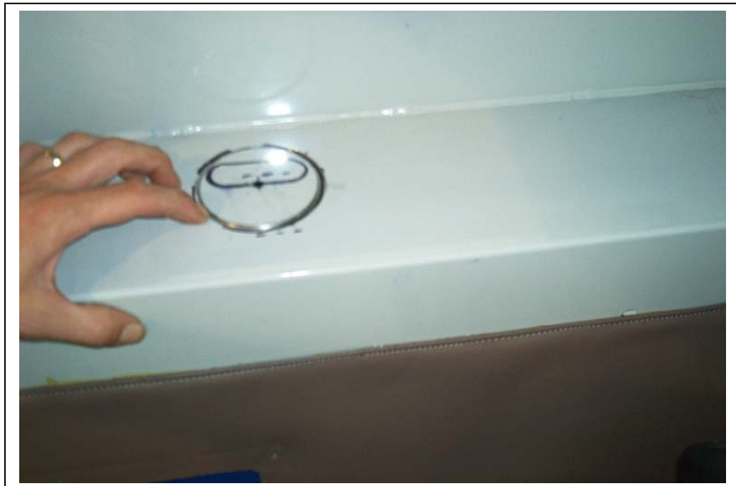
Using template provided, drill holes through to engine compartment to run A/C lines and electrical.
